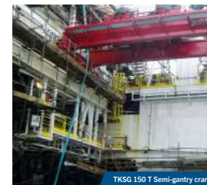
TKSG 150 T SEMI-GANTRY CRANE - Hydraulic drive by ringline system - Two trolleys for BOP handling
